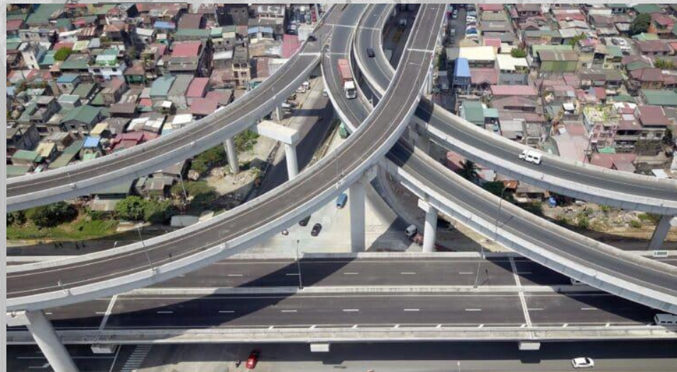
66% of the construction of the España to Sta. Mesa section has been completed as of Oct 2023
